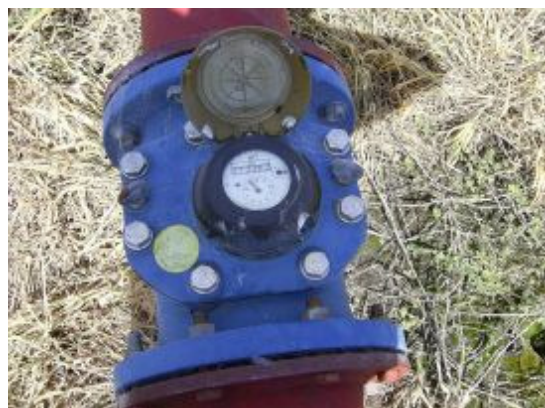
A water meter tracks irrigation use accurately
