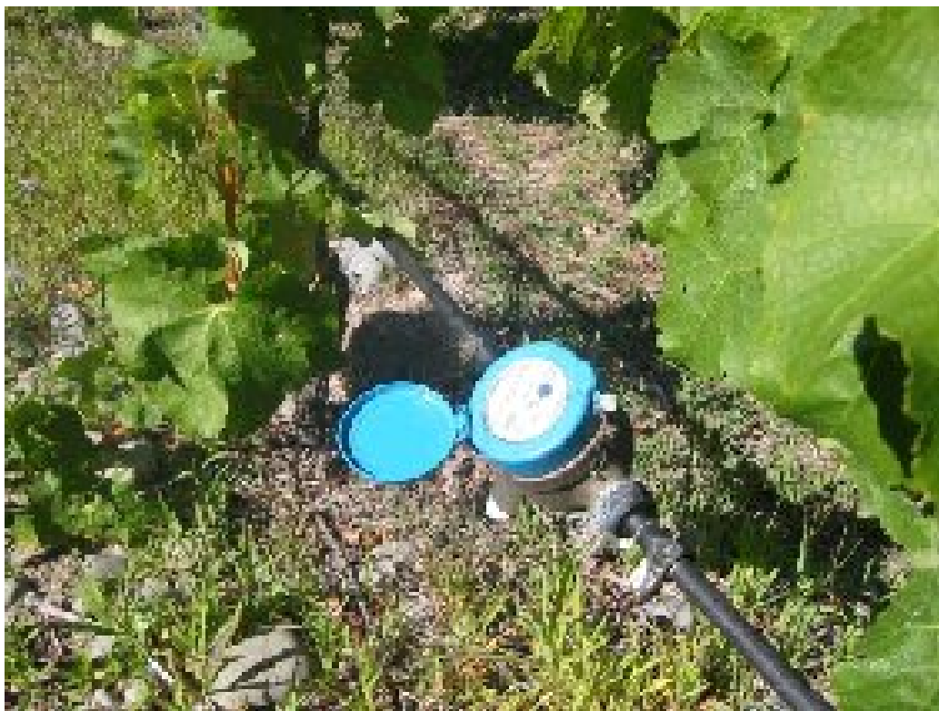
Figure Three Water meter
