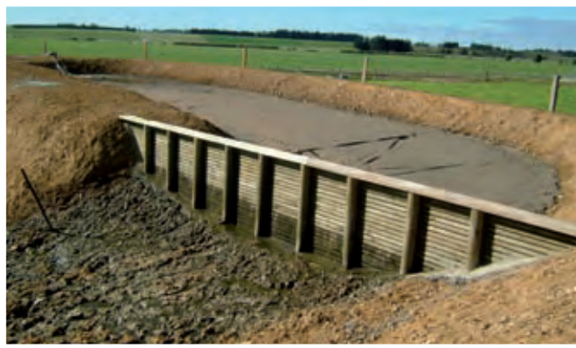
Sludge pond and weeping wall - Photo Courtesy Scandrett Rural
