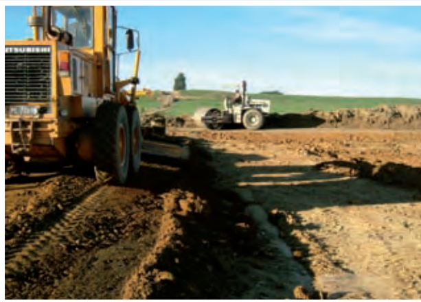
Compaction of embankment during construction of storage pond Photo Courtesy Scandrett Rural
