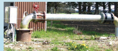
Meter too close to elbow.
